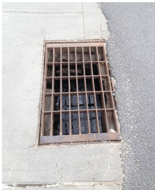
Full stormwater inlet after minimal rainfall
