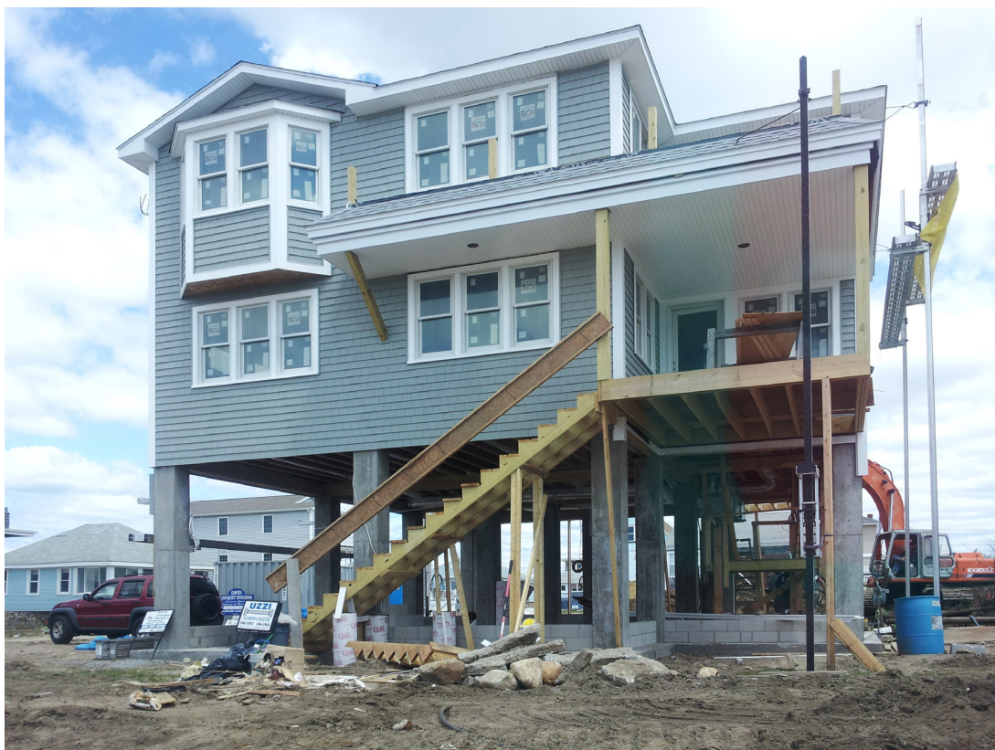
An example of a typical rebuild. Houses are raised to FEMA standards and sometimes built-out larger than the house they replaced.
