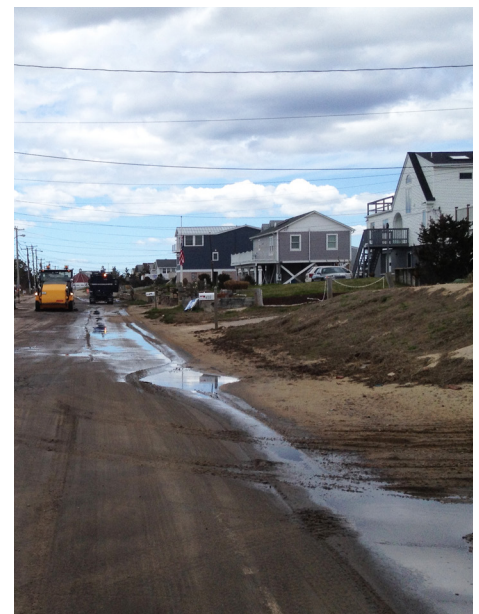
Pooling of water on impervious roadway
