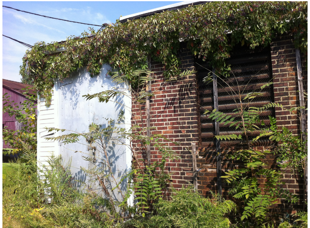
Many structures in the study area are overgrown or underused, but carry significant potential for adaptive reuse
