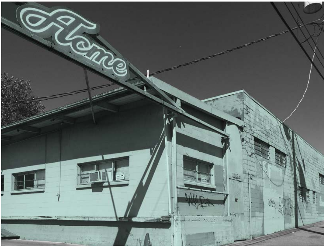
Many structures throughout the district are in need of revitalization
