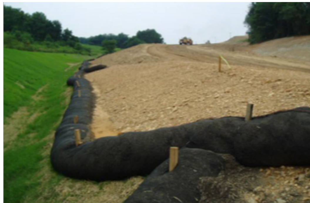
Compost and Compost Filter Sock Used for Soil and Sediment Erosion Control. Images from PennDEP. (2012). Erosion and Sediment Pollution Control Program Manual.
