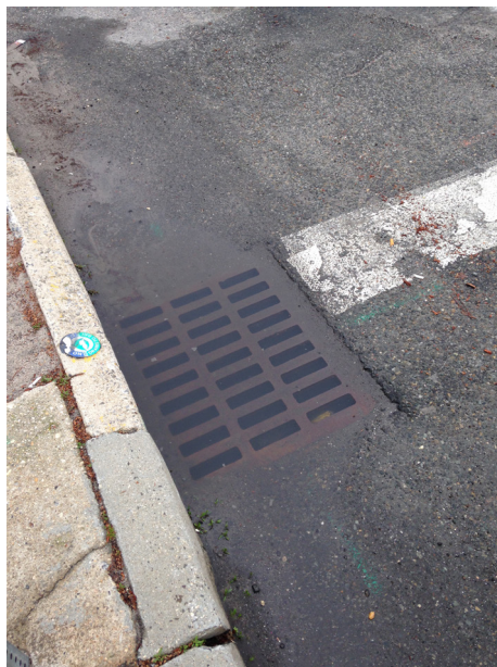
Backed up stormwater inlet during minor storm
