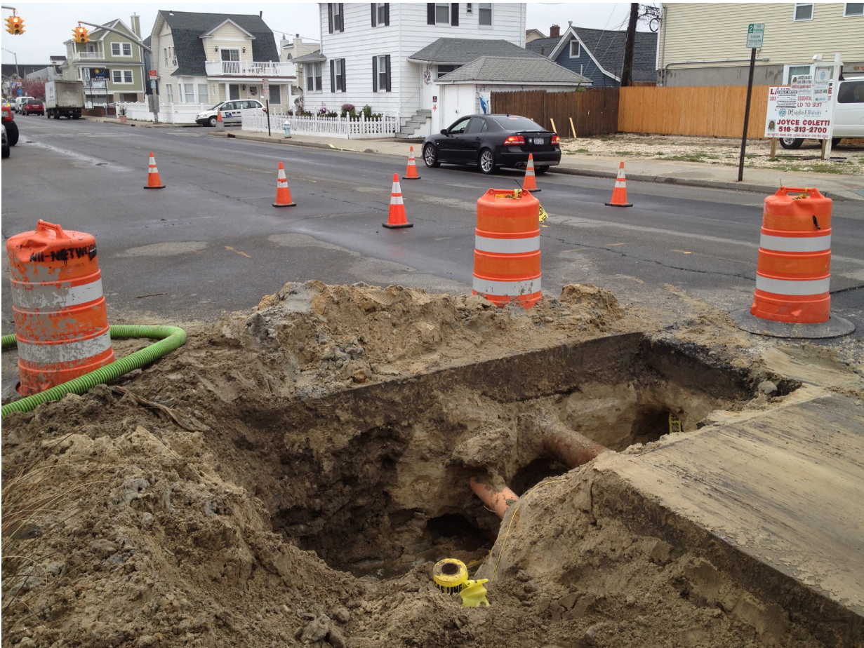
Damage caused by Superstorm Sandy included major infrastructure disruption due to the sandy foundation of the West End
